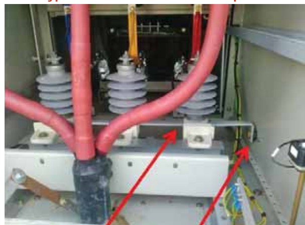
Earth bus of LA. (insulated supports) Earth bus goes out of panel through an insulated rubber bushing
