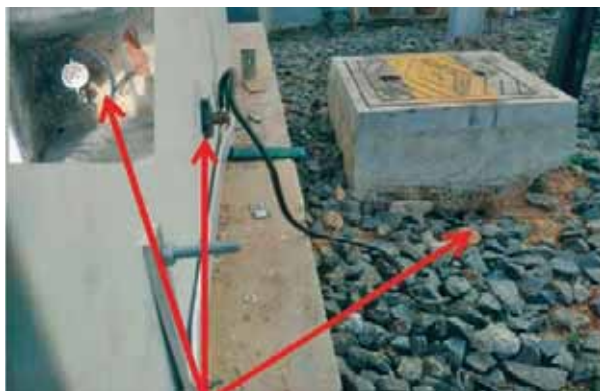
Earth bus goes out of panel through an insulated rubber bushing
